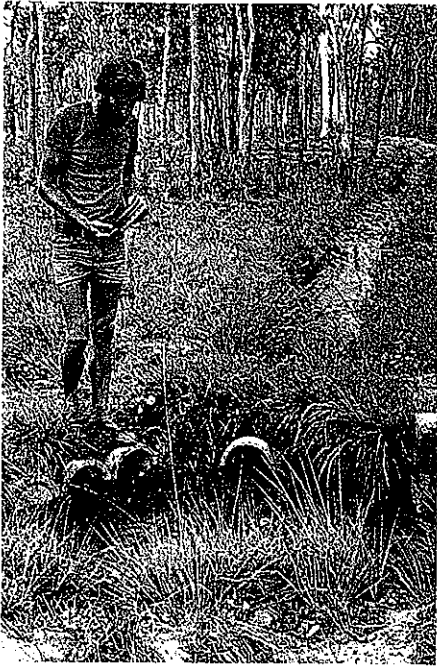
43. MALANDA, QUEENSLAND, AUSTRALIA. BOB KINGWELL has devised a simple manifold to lead water in 3 directions from a head drain; pipes are plugged or opened to allow flow in channels, using simple concrete plugs with rubber "O" rings.
